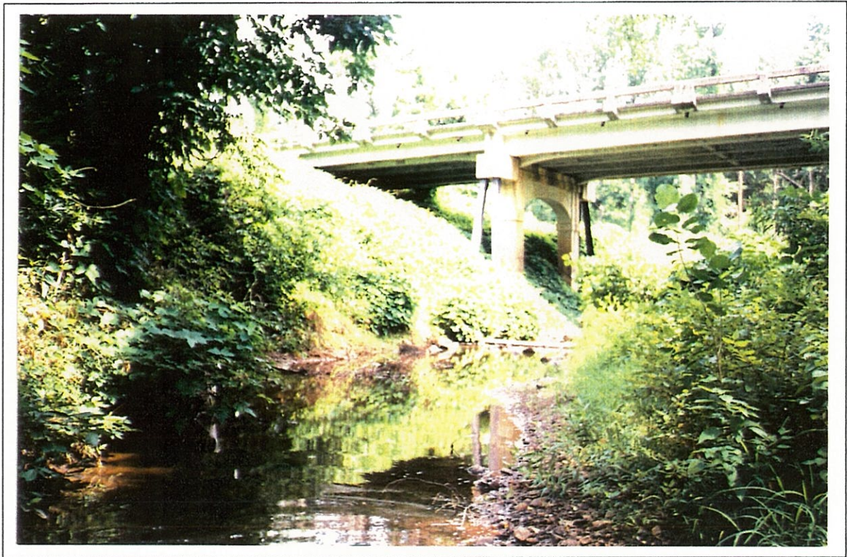
Figure 7. --Structure 124000900600 on Route SC 9, crossing the Sandy River in Chester County, South Carolina as viewed from the downstream channel (July 17, 1990).
