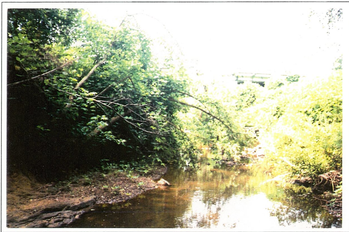
Figure 5. --Structure 124000900600 on Route SC 9, crossing the Sandy River in Chester County, South Carolina as viewed from the upstream channel (July 17, 1990).
