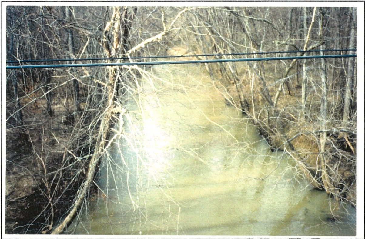
Figure 6. --Downstream channel as viewed from structure 124007200200 on Route SC 72, crossing the Sandy River in Chester County, South Carolina (January 28, 1991).
