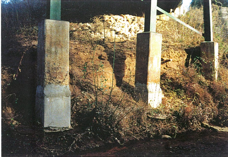
Photo 5: View of east bank - note erosion under encasement extensions for the piles of bent 2.
