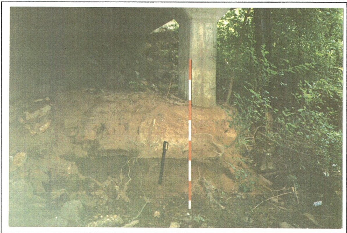
Figure 8. --Erosion of right bank at structure 124007200700 on Route SC 72 crossing Rocky Creek in Chester County, South Carolina (July 18, 1990).
