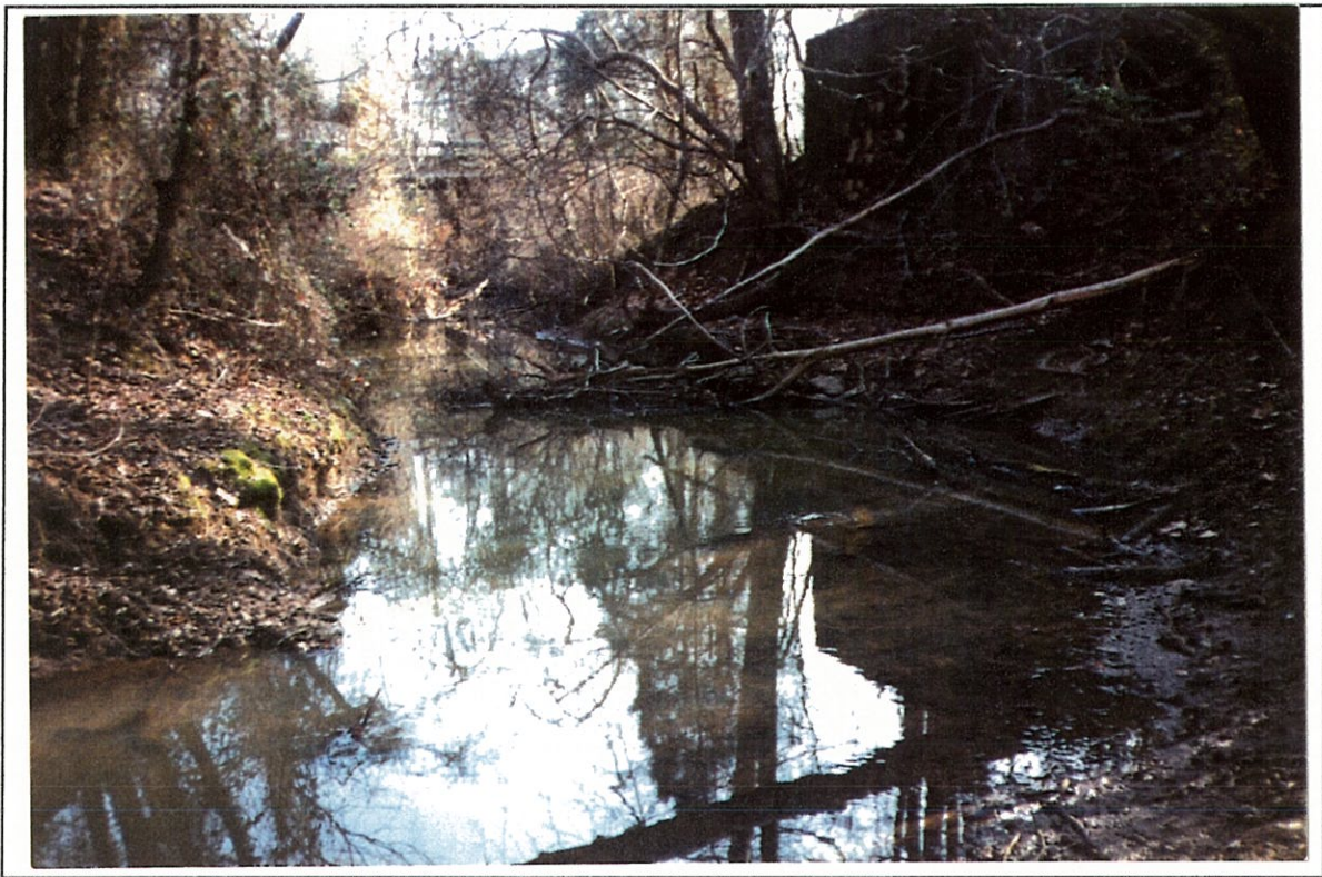
Figure 5. --Structure 124007200700 on Route SC 72, crossing Rocky Creek in Chester County, South Carolina as viewed from upstream (February 11, 1992).
