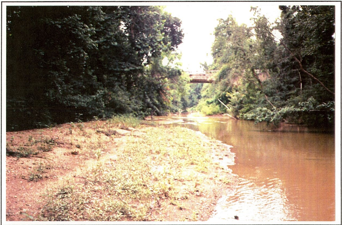
Figure 4.--Structure 124009700800 on Route SC 97, crossing Rocky Creek in Chester County, South Carolina as viewed from upstream (July 19, 1990).
