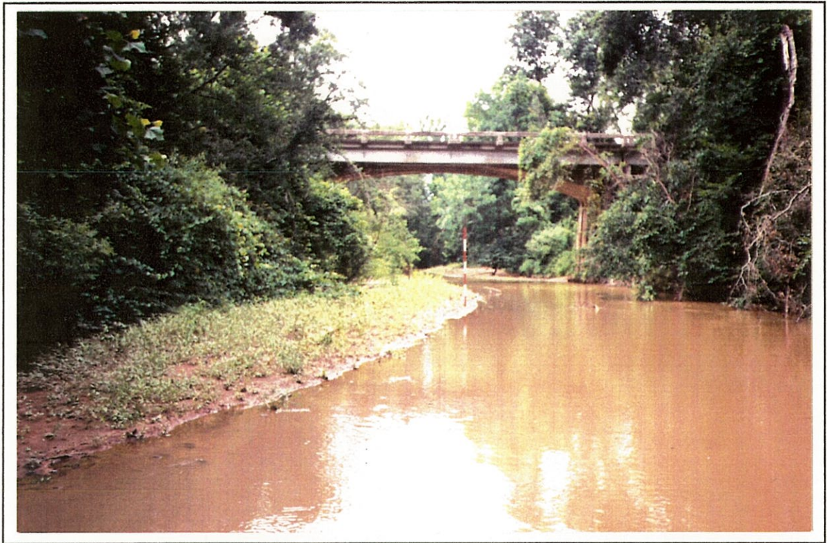
Figure 6. --Structure 124009700800 on Route SC 97, crossing Rocky Creek in Chester County, South Carolina as viewed from downstream (July 19, 1990).
