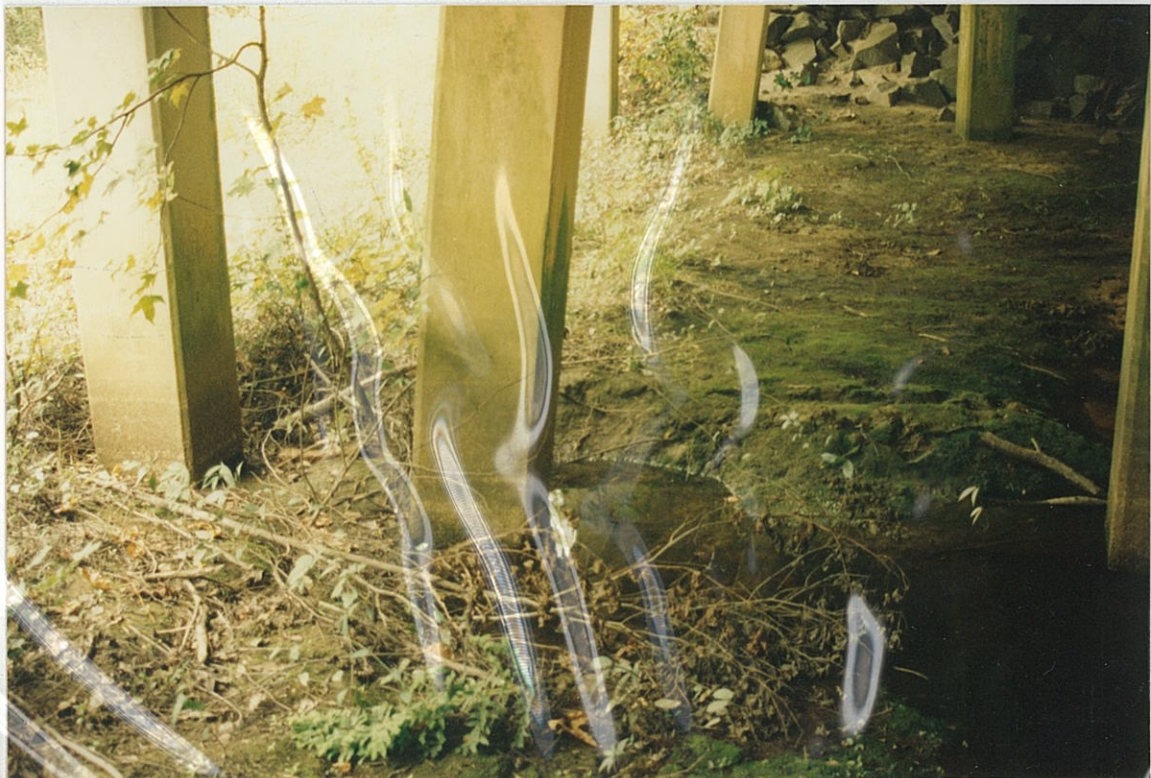
(6) Scour Hole at Bent 3
