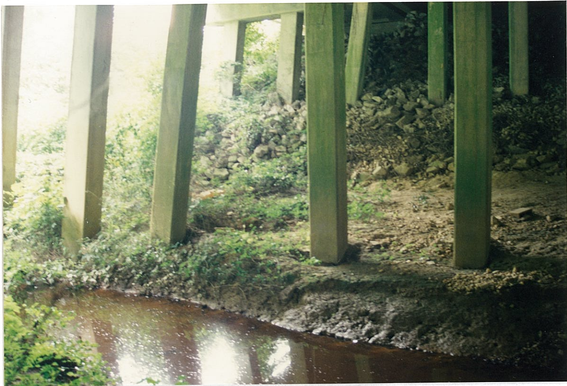
(9) Upstream side of End Bent 1
