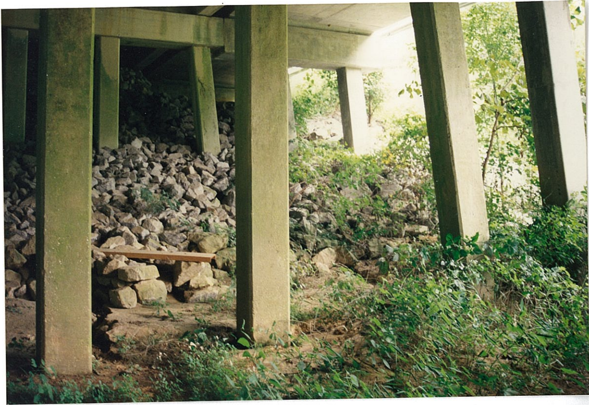
(7) Upstream side of End Bent 2
