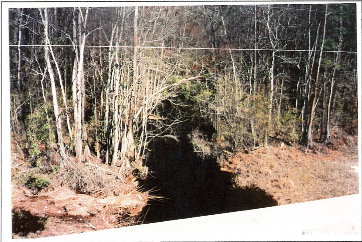
Figure 5.--Downstream channel as viewed from structure 132005200200 on Route US 52, crossing Juniper Creek in Chesterfield County, South Carolina (March 16, 1994).
