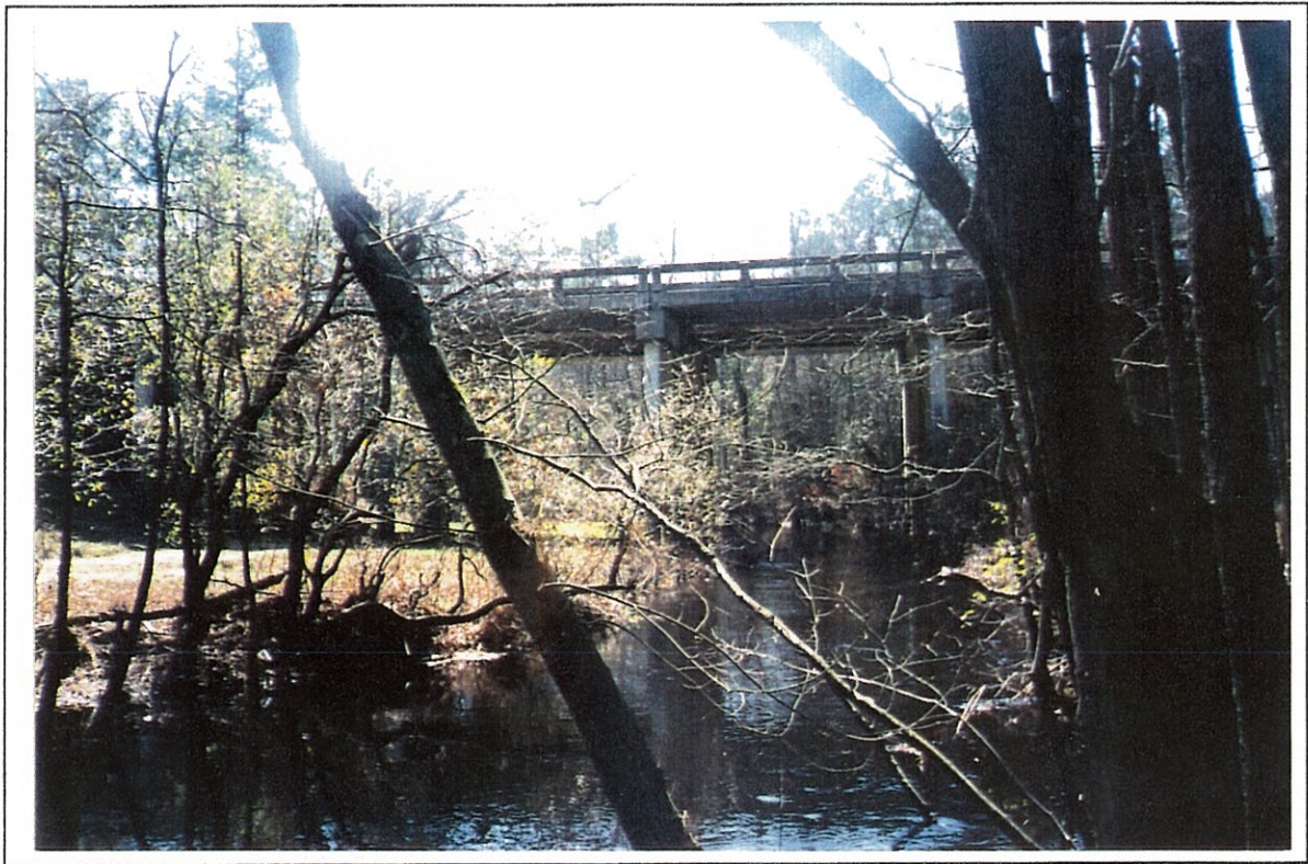
Figure 4.--Structure 132005200200 on Route US 52, crossing Juniper Creek in Chesterfield County, South Carolina as viewed from the downstream channel (March 16, 1994).
