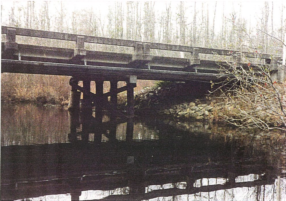
Photo 4- View of north abutment and bent 2 looking upstream. Riprap is in good condition.
