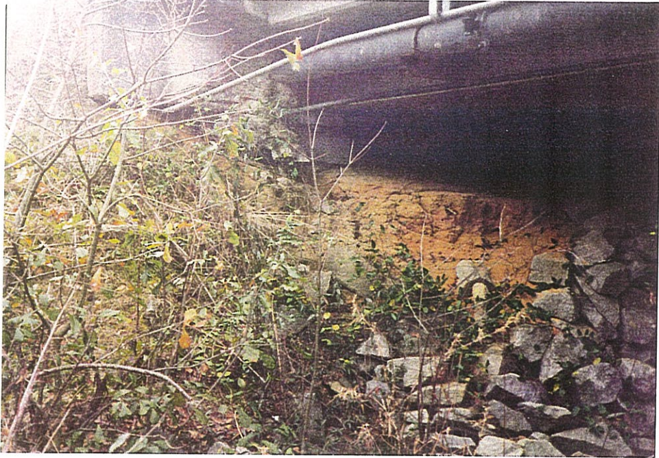
Photo 3- View of south abutment. Riprap is in good condition. Note erosion under the pile cap due to roadway runoff.
