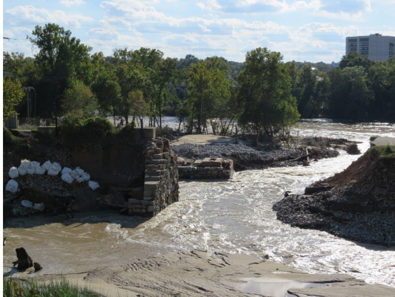
Figure 9. Columbia Canal breach Photo Source: Wes Tyler, SC Climatology Office
