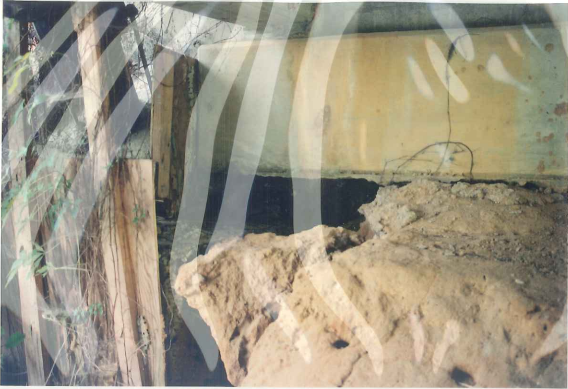
(5) Exposed pile, upstream side, End Bent 1
