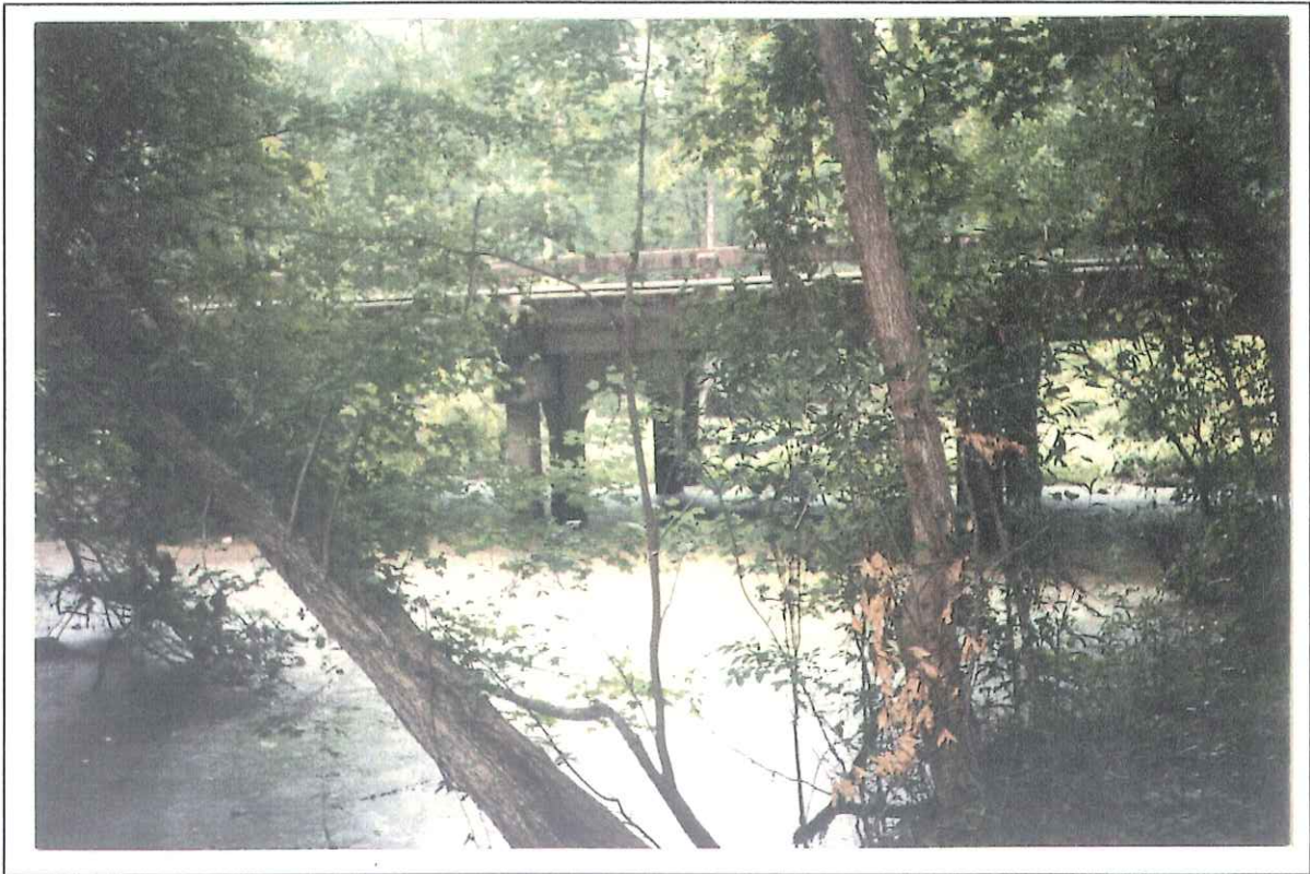
Figure 4. --Structure 182007800100 on Route US 78, crossing Cattle Creek in Dorchester County, South Carolina as viewed from the upstream right bank (May 24, 1990).
