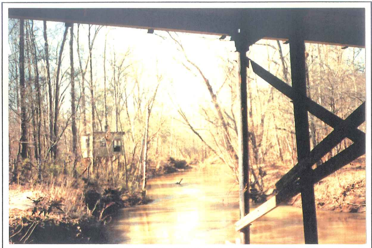
Figure 5. --Downstream channel as viewed from structure 194023000500 on Route SC 230, crossing Home Creek in Edgefield County, South Carolina (January 22, 1991).
