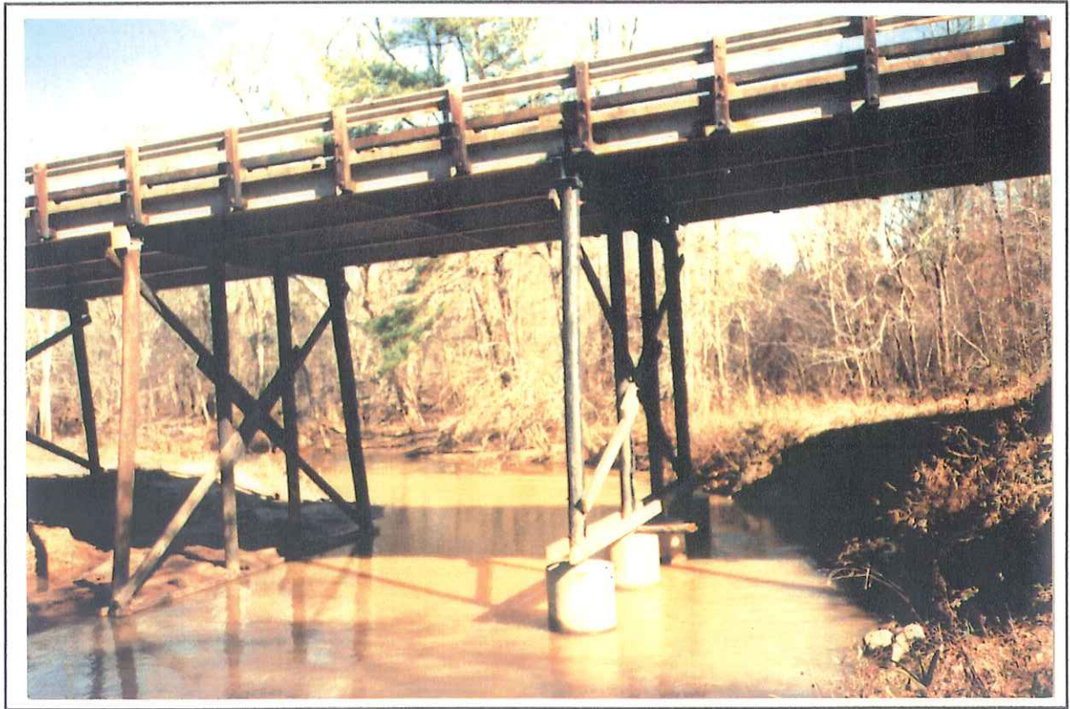
Figure 4. --Structure 194023000500 on Route SC 230, crossing Home Creek in Edgefield County, South Carolina as viewed from the downstream left bank (January 22, 1991).
