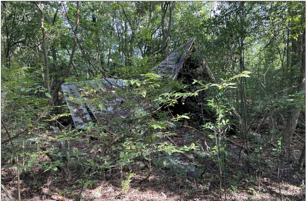
Figure 5.36 Collapsed structures north of Tunnel Road showing shed facing north (top) and barn facing northwest (bottom).
